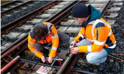
Predictive maintenance at rails (wired)
