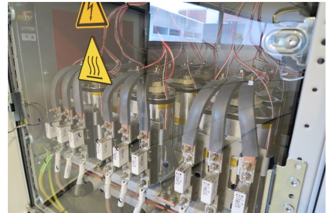
Capacitor bank for the grid-side filter
