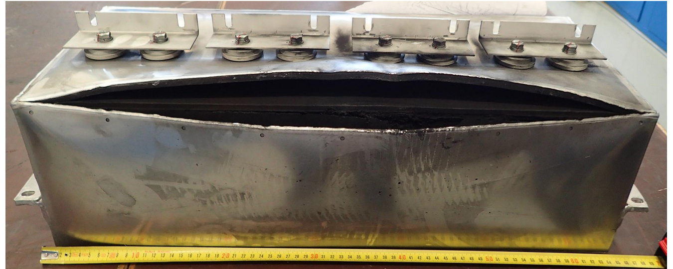
11 mF Film Capacitor Bank after Failure [2]
